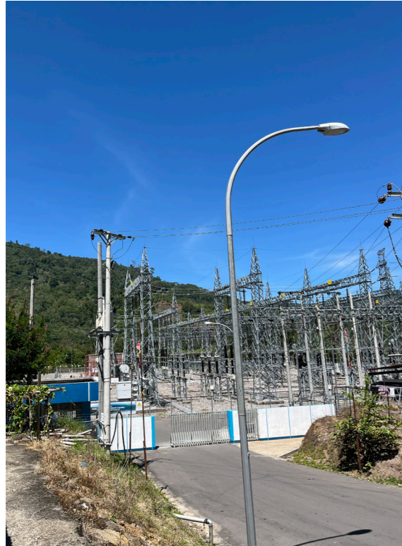
The Silih Nara Hydropower Plant in Central Aceh. (Photo: ACCI USK)
